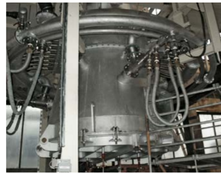
Lower part with gas burners
