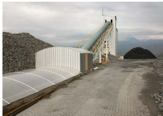
Conveyor to raw material bunkers
