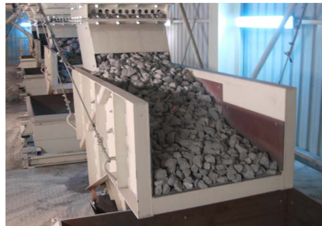
Batch feeding system
